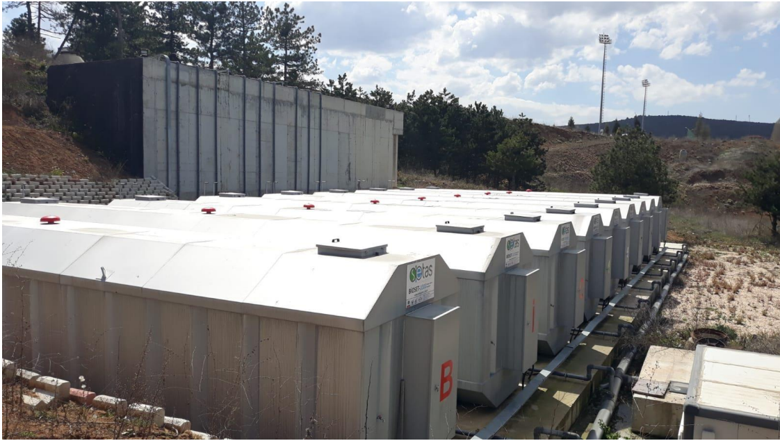
WWT Units, six packs total 900 m 3 /day
